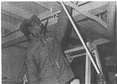
SA Phillips stretches high on a ladder to paint an inaccessible section of the overhead.
